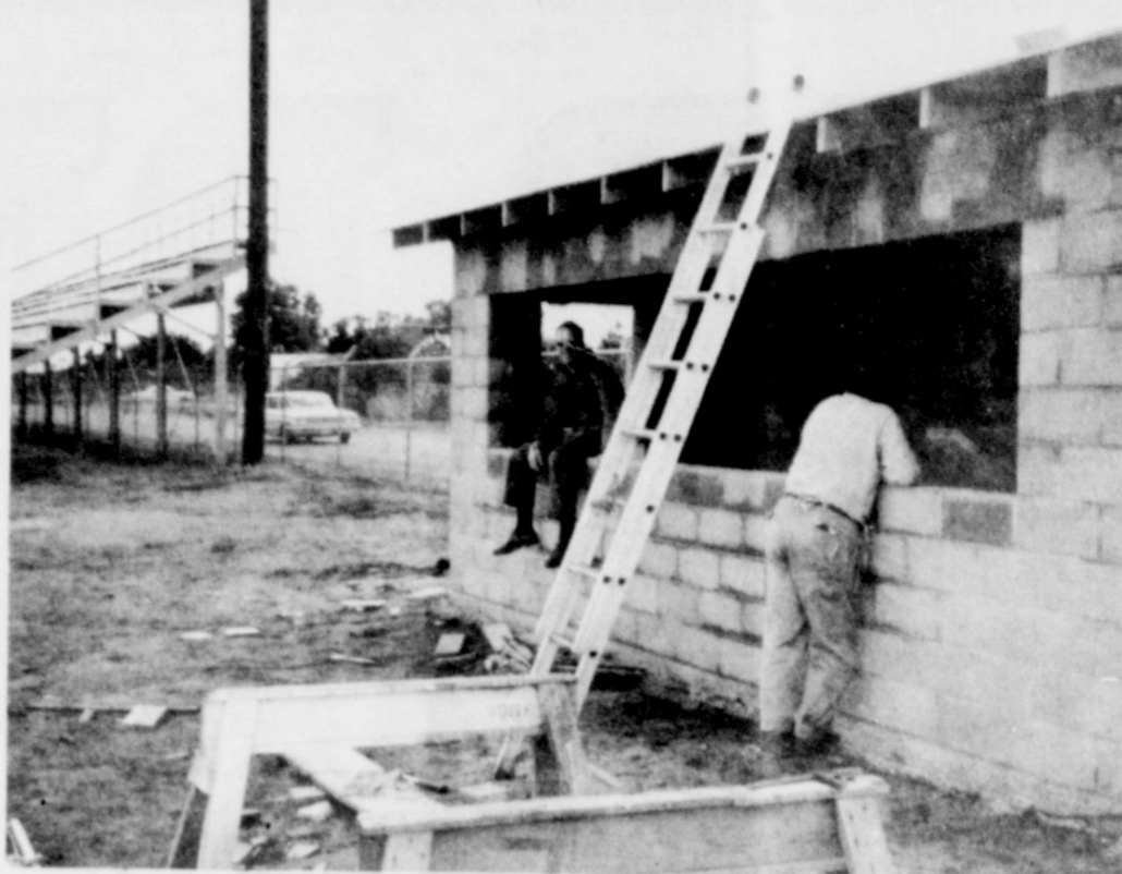
BUILD CONCESSION STAND - The Band Aids are building a new concession stand on the West side of the football field. Pictured here is the stand under construction with J. T. Miller and Robert Edwards supervising the construction. Proceeds from the stand will go to the Band. (Staff Photo)
