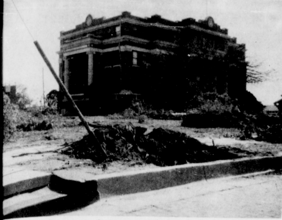
Down come the trees around the Lynn County Court House as work begins preparing the lawn for re-seeding. The trees have been a part of the court house for several years. News Photo
