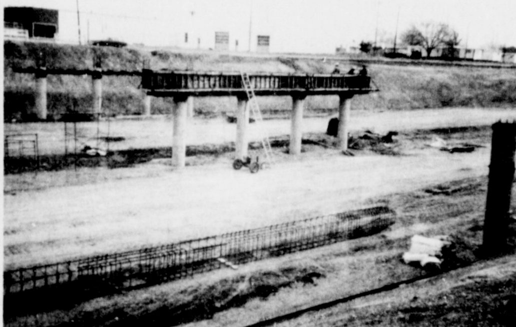
WORK IS BEING COMPLETED TO READY THE OVERPASS SUPPORTS FOR MORE CONCRETE AND STEEL. THE OVERPASS WILL GIVE EASY ACCESS TO BUSINESS AREAS EAST OF THE BYPASS. STAFF PHOTO
