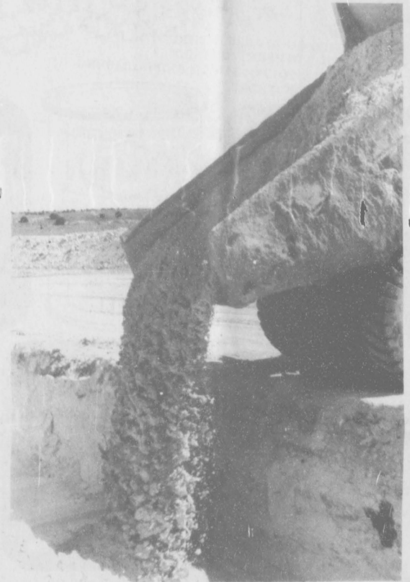
This was one of many truckloads of sand that was being dumped into the core of the dam last Thursday. Workers are still busy finding the right grade of sand for the project.
