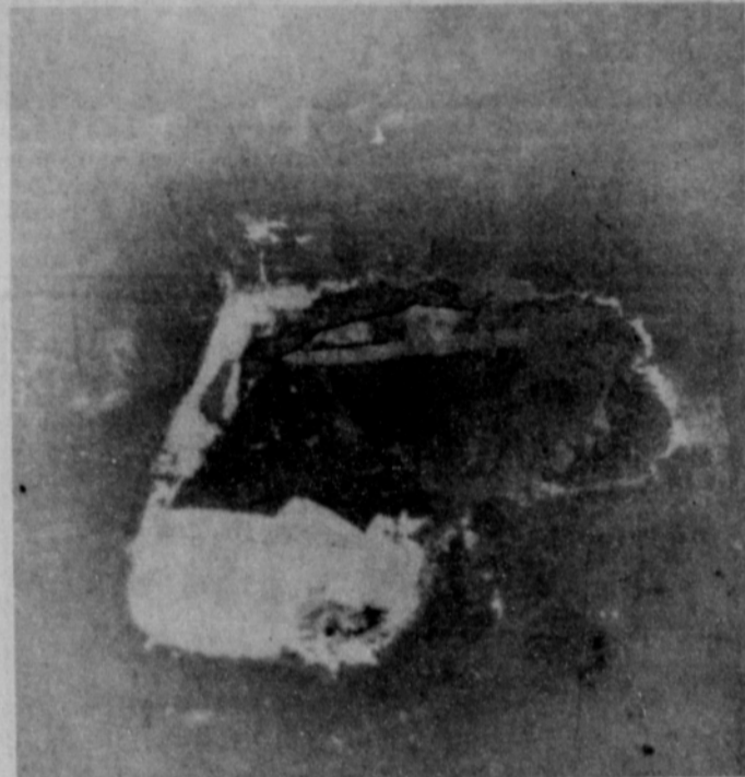
PLASTER OFF - The plaster is off a hole in the cement part of the wall in junior high. It is repair work of this nature that is needed in the building.
