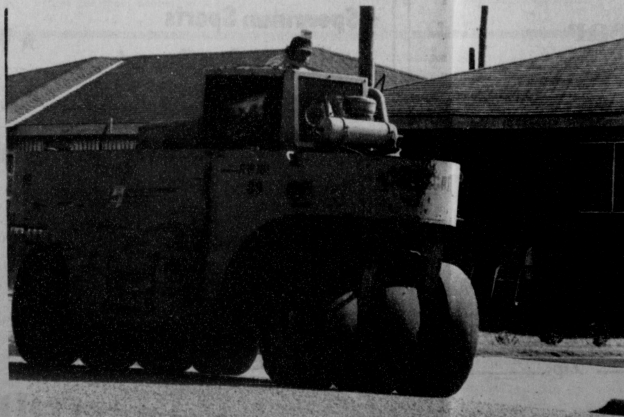
SEAL COATING OF SPEARMAN STREETS came to an end Friday as crews packed down the special tar and gravel mixture on city streets. The one-week operation
