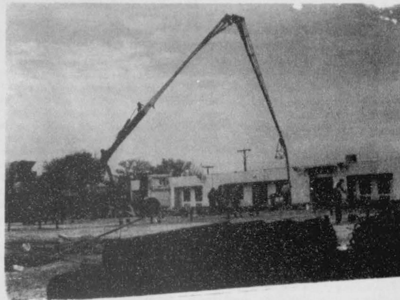
Construction going strong. This is the scene at the Hansford Manor as they are building the new addition.
