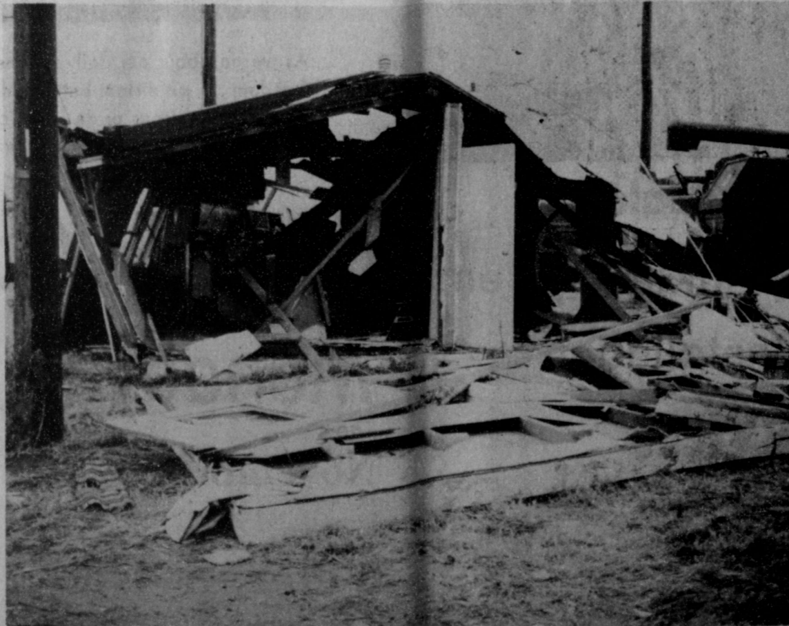
The Spearman Fire Department answered a call this week, at Spearman Super Service, as this building pictured "exploded" apparently from a gas leak. No one was in the building, and no one was injured. The small office-type building is located in front of Super Service.
