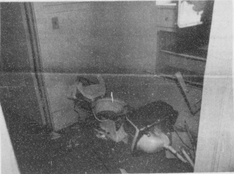
The bathroom at the Lasater ranch was destroyed.
