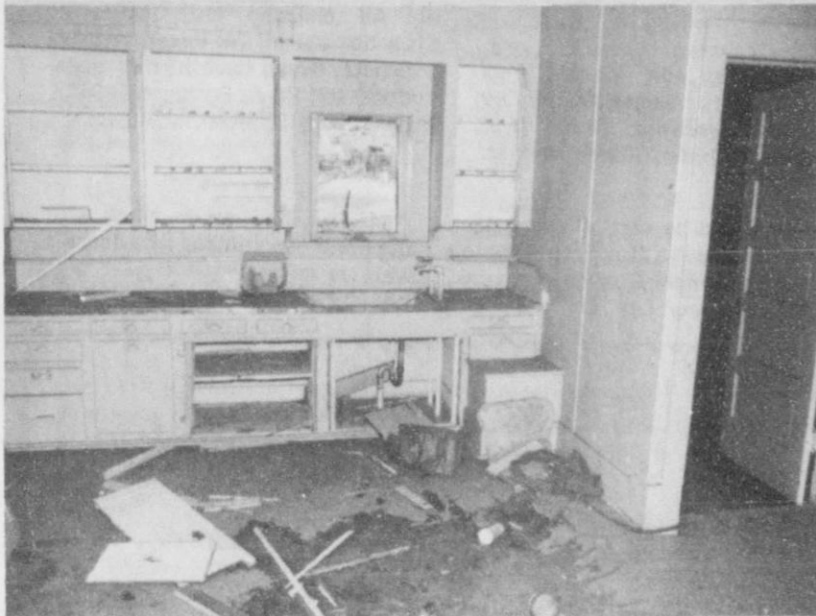
The kitchen at the Lasater Ranch was almost completely destroyed.
