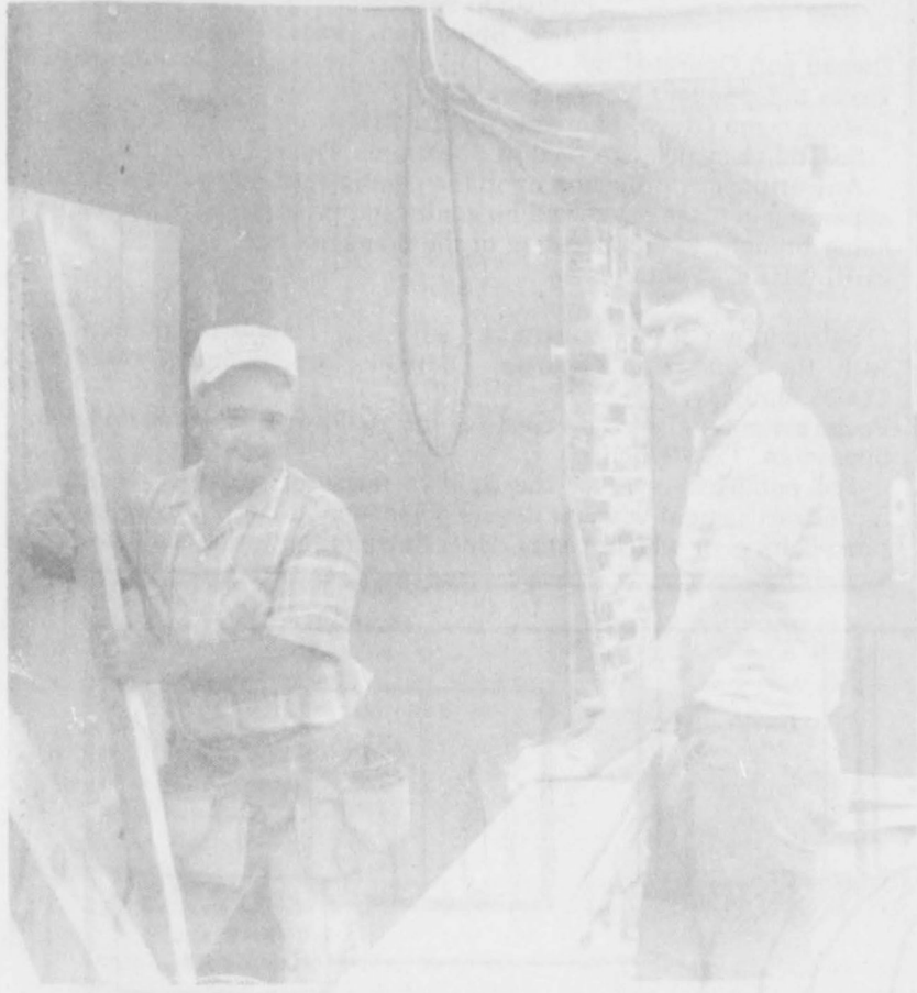
These two men are putting the final touches on the Pizza Hut construction work. Friday, Darryl Rucker [left] and Rocky Grant of Grant Construction were building a fence around the cooling system. This job completed the remodeling work of the restaurant.
