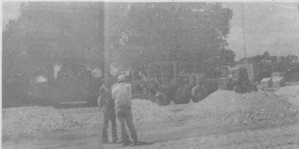
The Hansford Manor is soon to have a new parking lot. Workers from the city of Spearman are constructing the parking lot and expect to be finished
