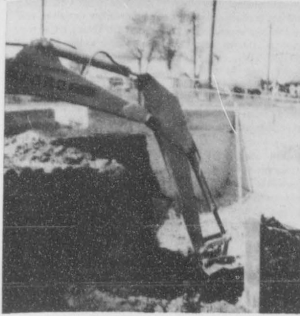
This picture shows the big machinery used recently to excavate the basement for the addition to the Stationmaster's House Museum. The work has been completed and already Preston and Archie Smith have the cement poured and the moving is ready to go. The Museum Board wishes to thank these fine men for their donated time and machinery.
