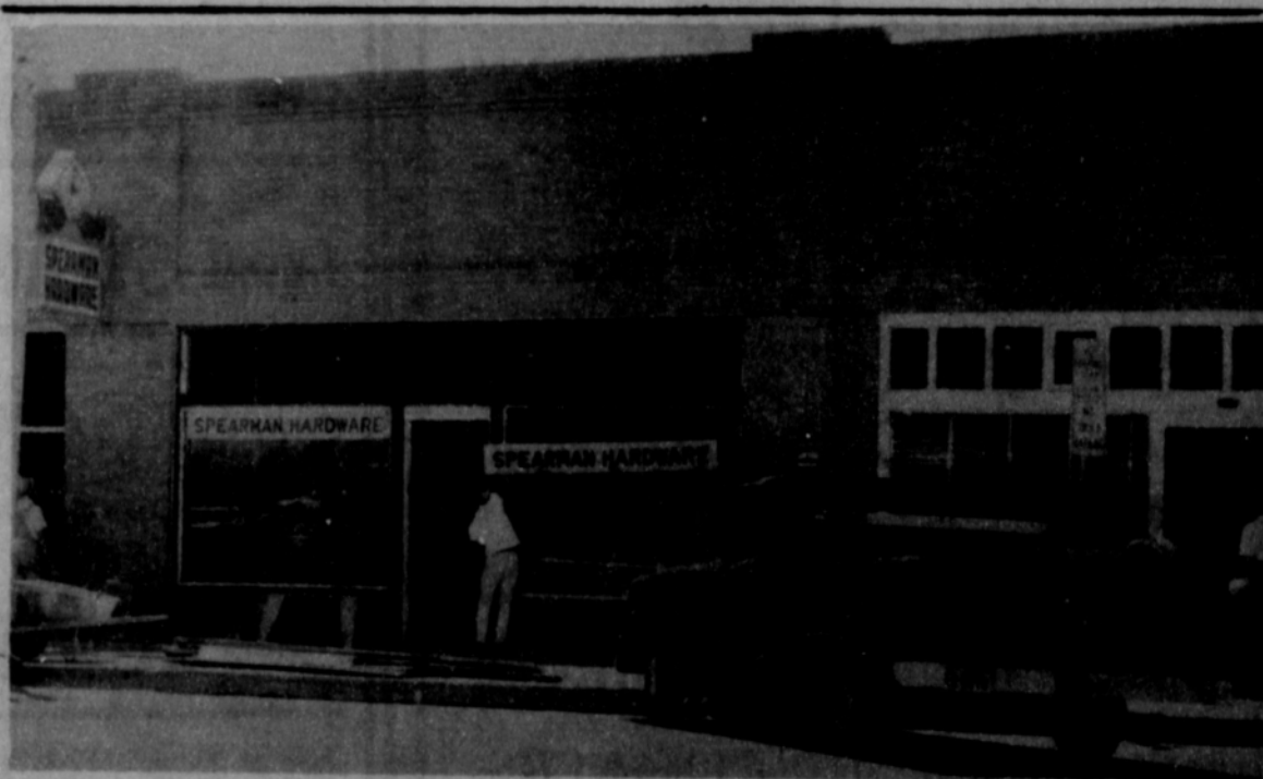
NEW FRONT--Glassworkers remove the windows from Spearman Hardware in preparation for installing a new front. Joe Trayler Ford also got a new front in the remodeling work. --Plainsman Photo.
