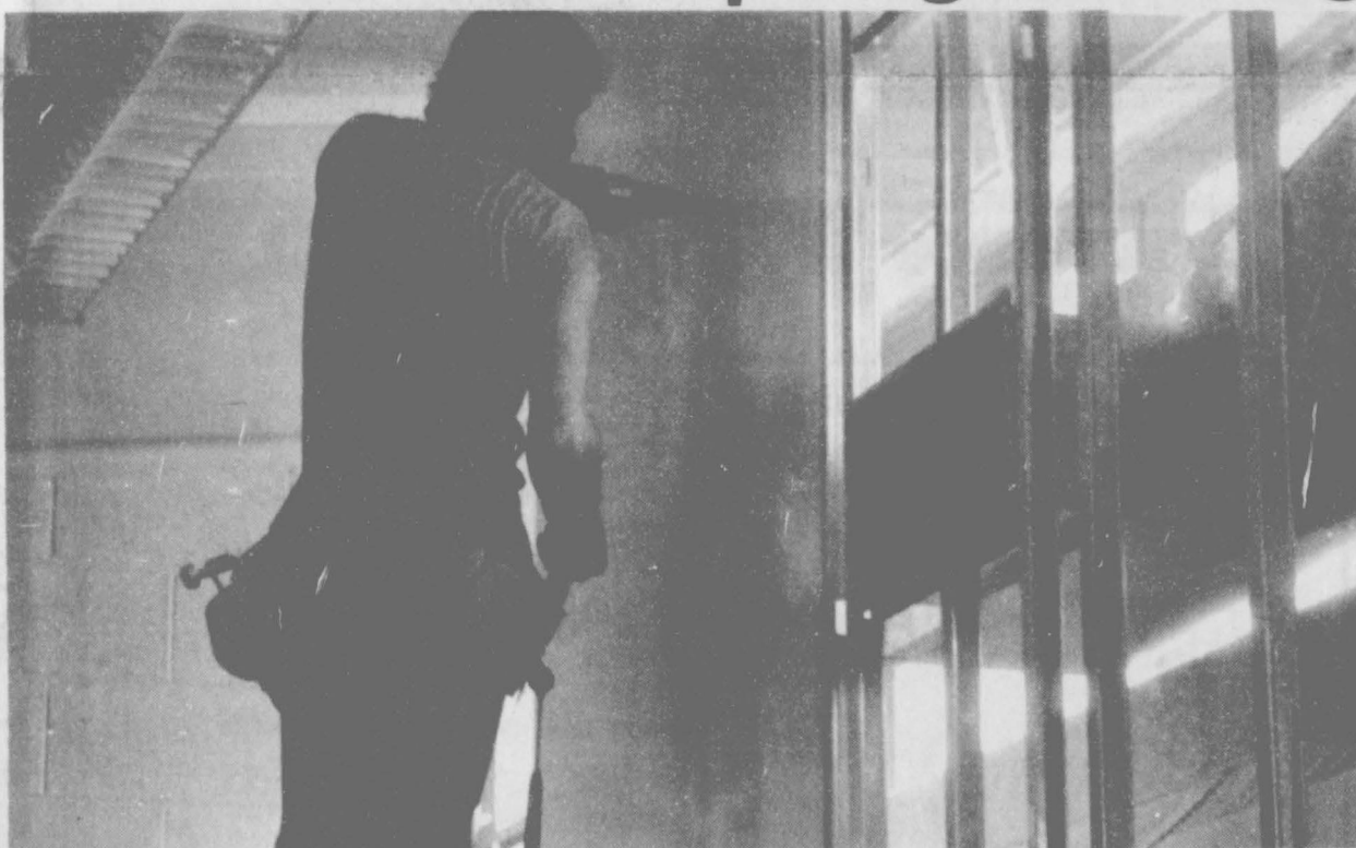
Shown here, David Nobile, one of the construction workers doing work on the Spearman Elementary School. Here he is putting sheetrock up over the new
