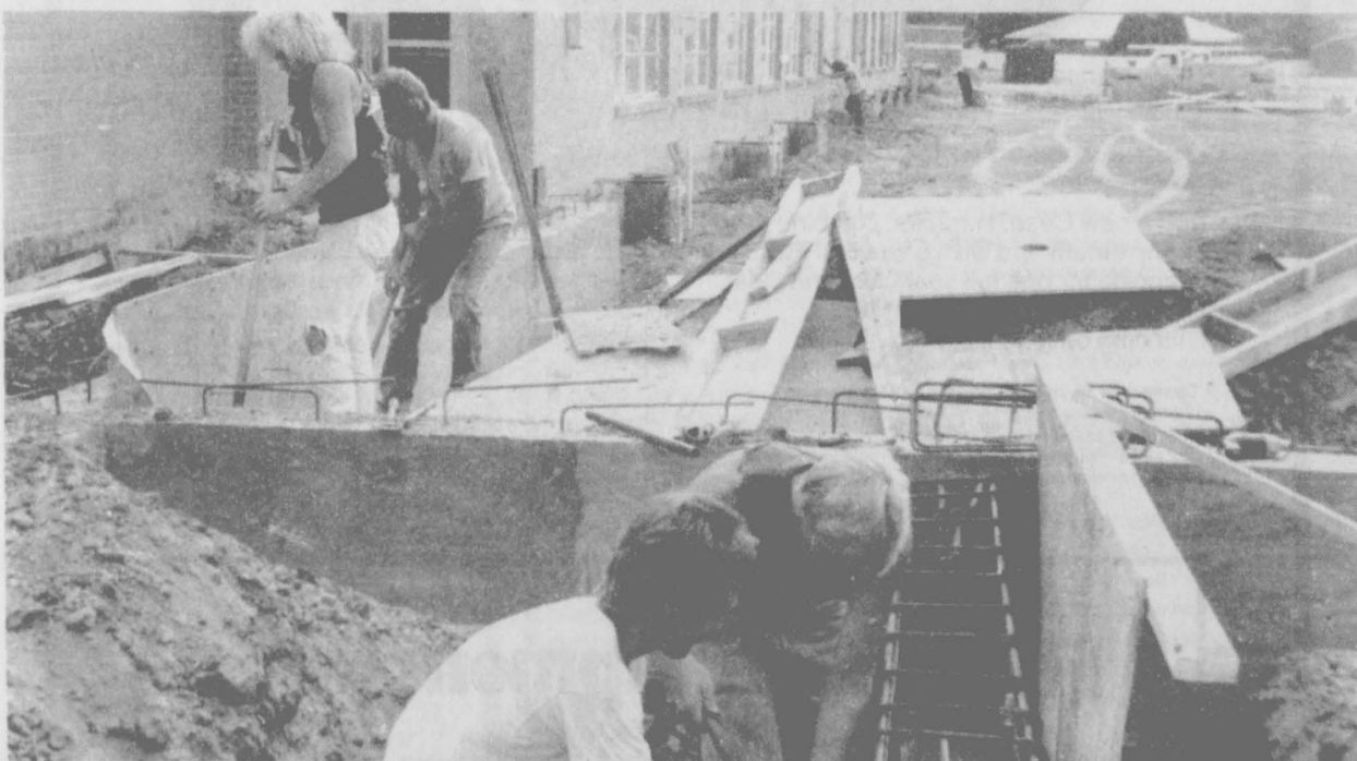
Work is still going steady at the Spearman school. These men are putting in steel supports that will be the beginning of the walls for the additional classrooms. The men couldn't take the time to give
