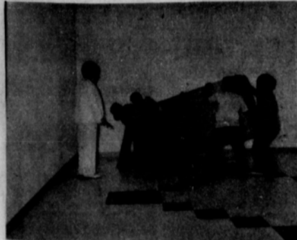
Mrs. Hutchison and Jr. High work crew install cabinet in one of the new rooms which once was the old Jr. high gymnasium.
