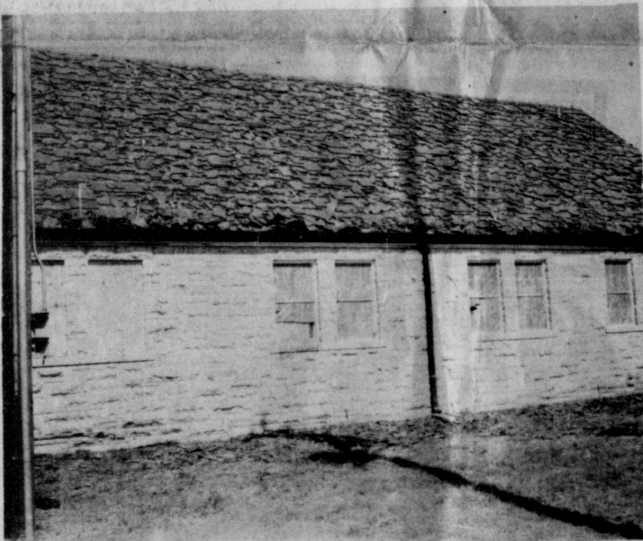
ROOF RUINED -- A section of the hail-battered Oslo church.
