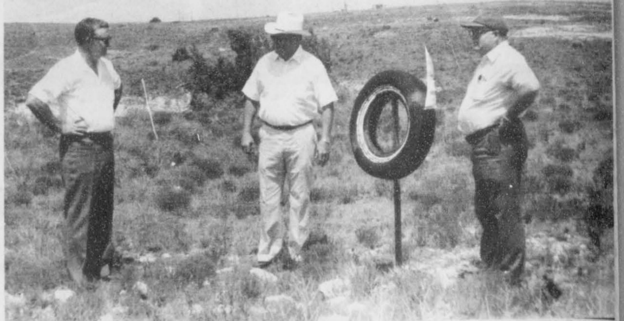
JACK OAKES, JOHNNIE LEE, and DWAYNE SMITH OF KRDF were on hand at the dam site Thursday of this week. The tire marks the spot where the dam will start on the East side of the breaks, located 10 or 11 miles north of Spearman.
