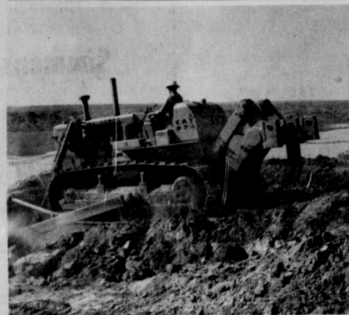
Fritch City Mayor Dick Hatfield tries the controls of big earth moving machinery . . . to be used in constructing the new road from Fritch to Lake Meredith.
