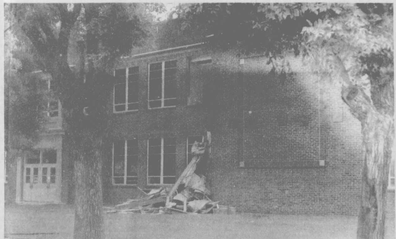
The Spearman Junior High School is starting to show the efforts of the wrecking project done by a crew from Oklahoma.
