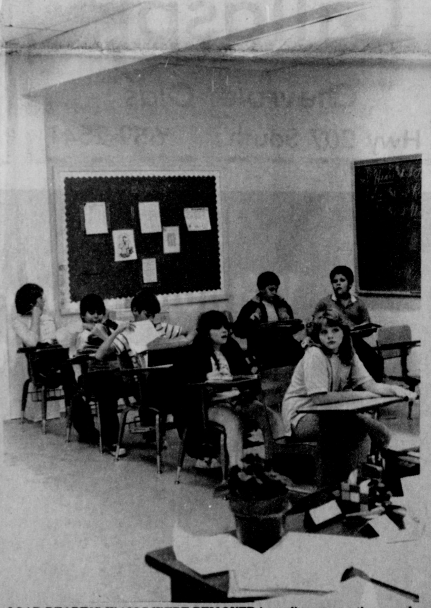
LOAD BEARING WALLS WERE REMOVED in earlier renovations, such as the one in this picture of Wynette Mullins' fifth grade class at Spearman junior high. Structural cracks in the ceilings have been patched over. Voters will decide Tuesday whether to condemn the east wing of the building in a $2.185-million bond issue ballot.
