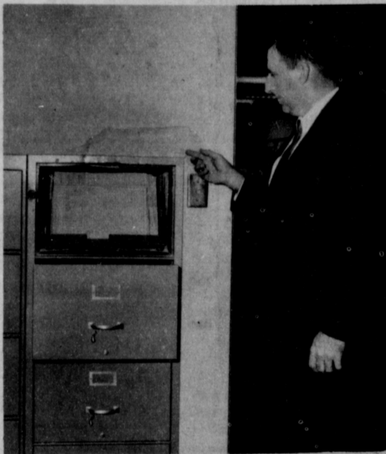
DAMAGE--Waka School Principal Bill Shelby points out the damage done by burglars to the wall and built-in file cabinet in the school over the weekend. Over $150 in cash was taken. Plainsman Photo
