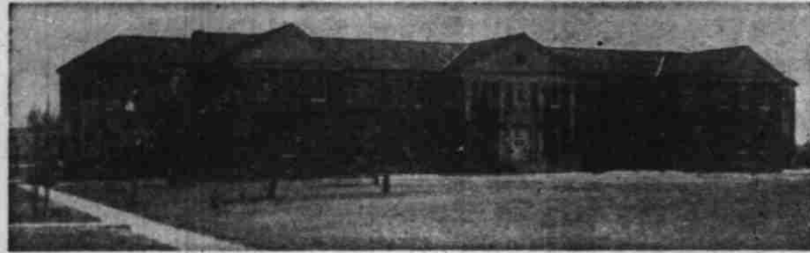
STUDY IN CONTRASTS—Consequences of poor planning are brought home by the "curbstone" in the above picture. This recently appeared in basement ward of Terrell State Hospital's main building. Settling of the earth caused half the building to rise and the other half to sink. Note doors had to be sawed off. Every building at Terrell has suffered from this phenomenon. By contrast, the picture below shows how a hospital building should look. This is a well designed ward at Big Spring State Hospital. Six more of these structures are requested in building plan now before legislature.
