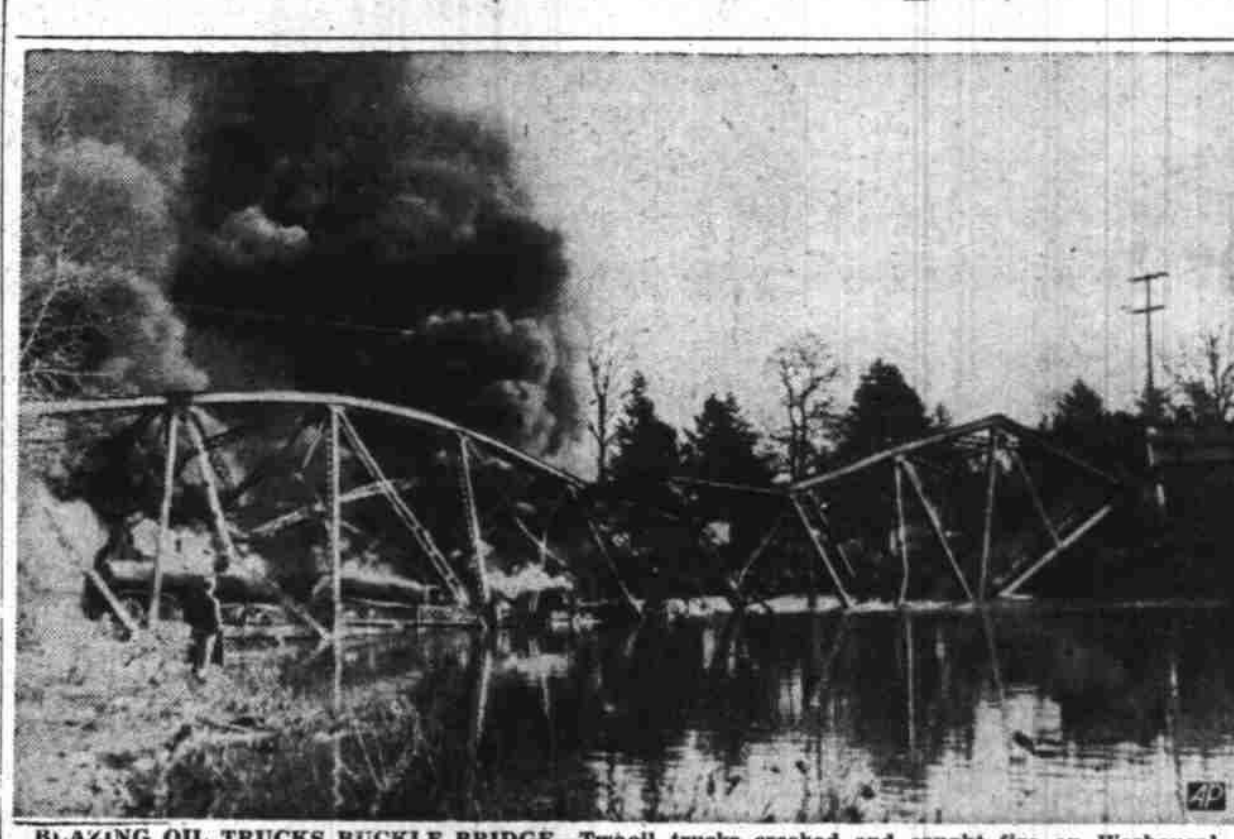
BLAZING OIL TRUCKS BUCKLE BRIDGE—Two oil trucks crashed and caught fire on Washington bridge at Vancouver, Wash. Intense heat caused the 220-foot steel structure to collapse closing Evergreen highway along the Columbia River. (AP Wirephoto.)
