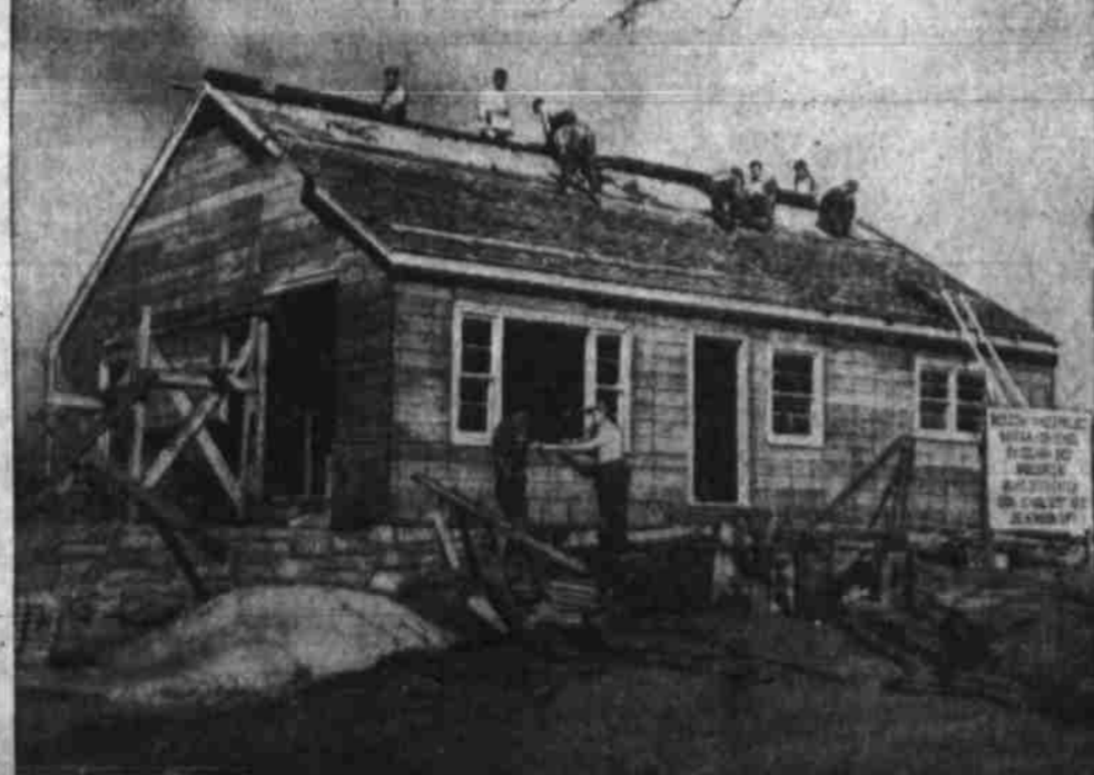
STUDENT PROJECT —Students in the building trades class of Raytown, Mo., High School, work on the six-room house with garage they are building as part of their class work.
