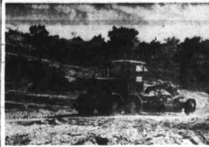
ROAD WORK —Nearly half of the expenditures by Howard county are for road maintenance, some construction and allied work. The county has more than 700 miles of dirt laterals. There are constant demands for opening new roads and relocating sections of old ones. Here a maintainer establishes road bed in a hilly section. (Jack M. Haynes Photo)
