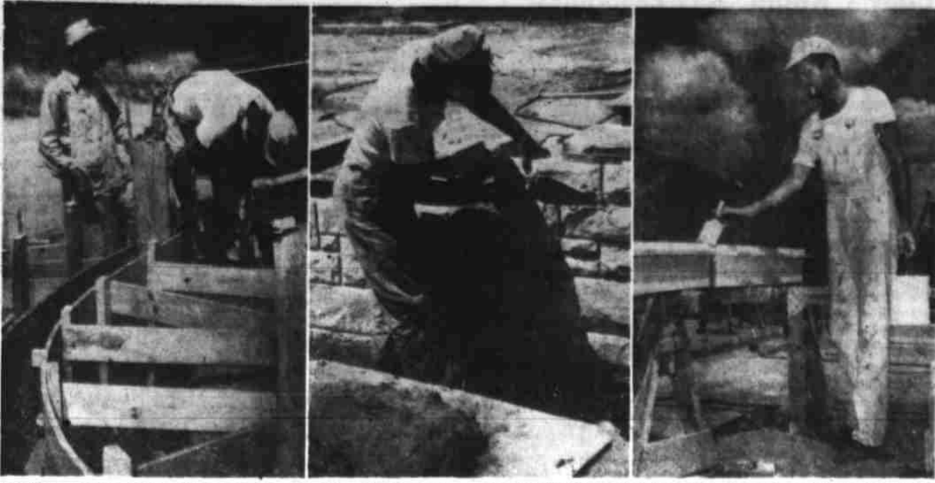
HOMES FROM HANDS —Whatever else goes into a home, it is the skilled touch of human hands that works the miracle. Scores of experienced craftsmen today fashion structures according to the most intricate designs, shape, finish and protect them for years to come. At left, workers set a sweeping form for concrete. Steel, behind one of the men, will bind and reinforce the mix for indestructibility. Center, A stone mason lays a tedious pattern of odd-size limestone with outside rough finish—a new and popular kind of outside wall. At right, a painter coats a frame before installation, part of the process to protect against the intense sun and wind of West Texas and its capricious and biting rains. (Jack M. Haynes Photos)
