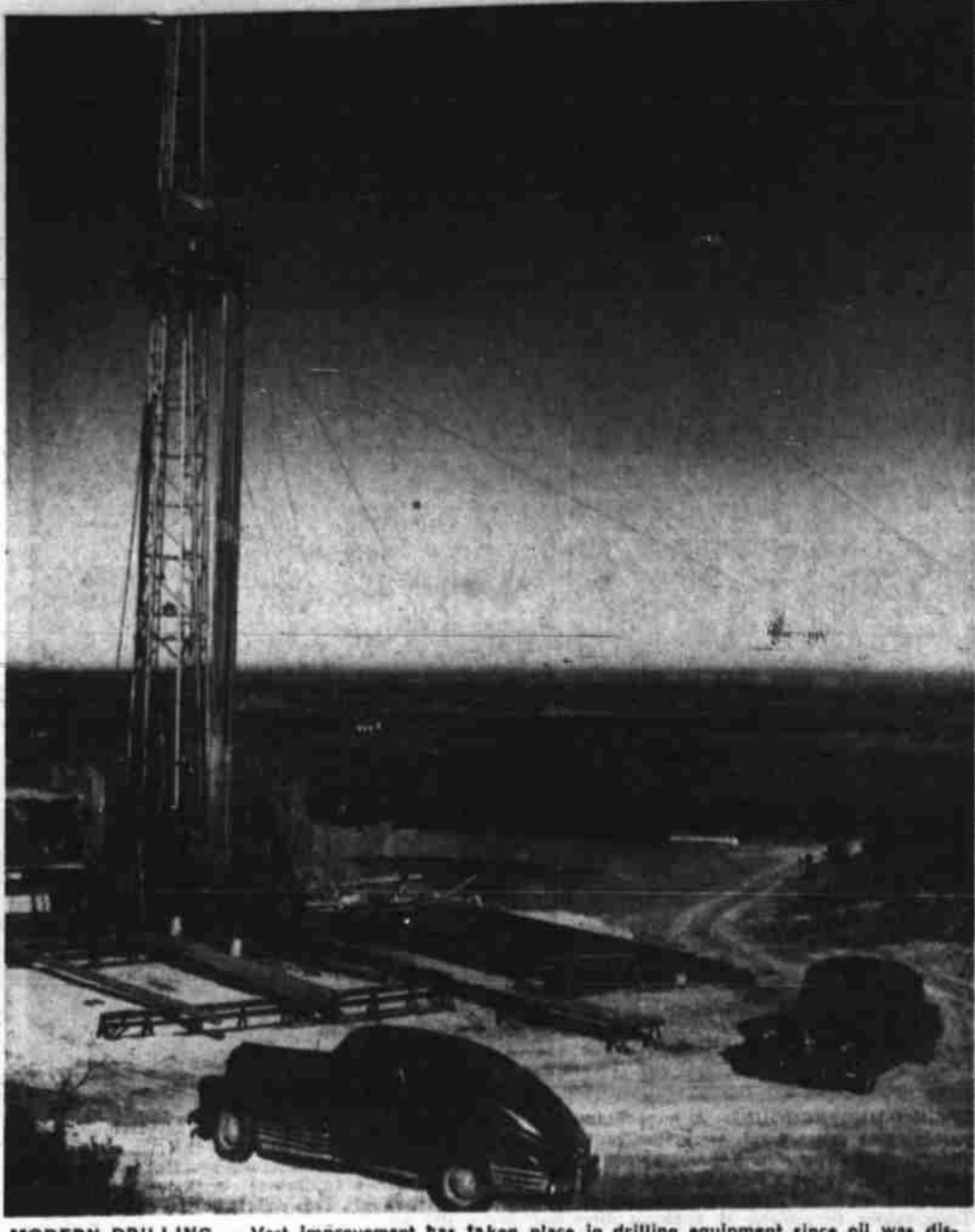
MODERN DRILLING — Vast improvement has taken place in drilling equipment since oil was discovered in Howard county 24 years ago. Typical of some of the smaller rotary rigs is the "jackknife" unit above. It is portable and may be moved easily to a new location. Moreover, it bores rapidly. Thirty years ago there was one rotary rig in this country, but it was a primitive affair. The rig above is on the Magnolia lease in the vicinity of where the first real commercial well for Howard county was completed in April 1926. (Jack M. Haynes Photo)
