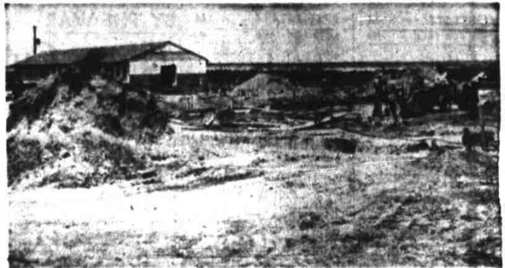
NEW HCJC PLANT IN MAKING —Workmen at Howard County Junior college's prospective new campus east of the city are nearing completion of foundation work for new buildings. Construction will "come out of the ground" in the near future. At the upper left of the picture is a frame building recently moved from the present HCJC site at the former Army Air Field. Building was moved by Busboom and Rath, general contractors, who will use it as a warehouse. It will subsequently be turned over to the college. The foundation will enable erection of an outside brick wall for the old building if the college desires. (Culver Photo)
