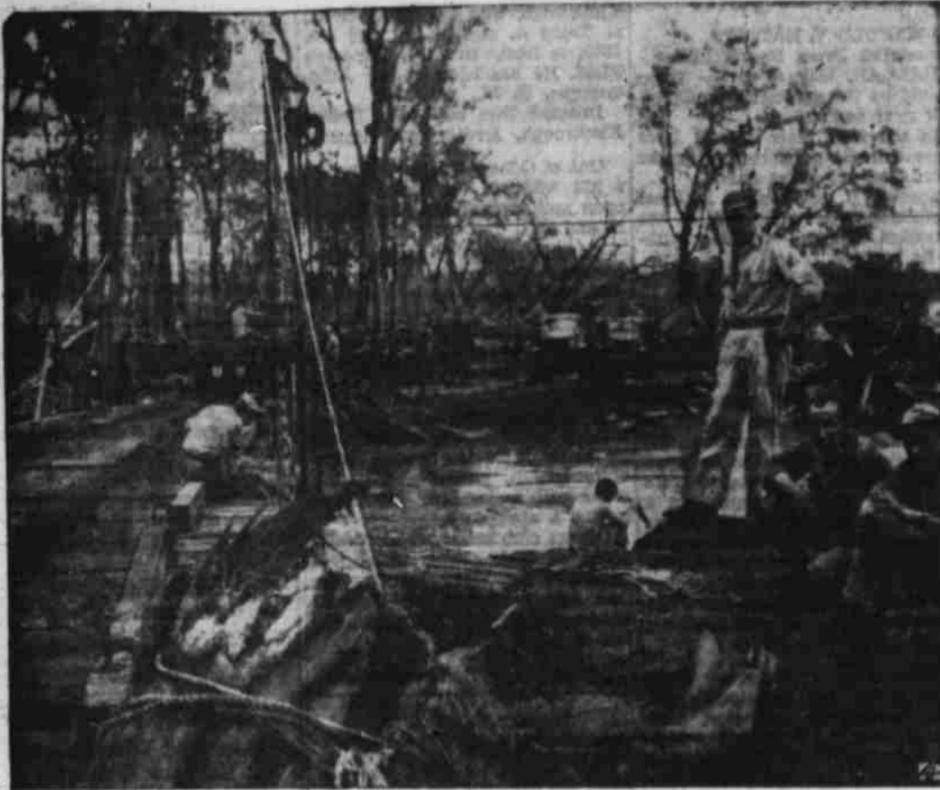
BRIDGE BUILDERS —As trucks wait to cross a stream on Cape Gloucester, Marine engineers finish a "Tubelox" bridge built to substitute for one washed out by a flood.
