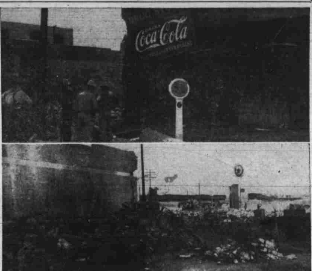
Here's what happened when fire broke out in the Adams Garage Sunday night at Coahoma. Below, ruins of the garage with car wheels tangled in other debris. Above is the front of the Nesbett Drug Co. which also was destroyed when the flames got out of control. Efforts to combat the blaze were hampered when Coahoma volunteer firemen ran over a plug and the hose supply was insufficient to reach from the next nearest plug. The Big Spring fire department sent over a truck and detachment of firemen and succeeded in bringing the fire under control without further damage.
