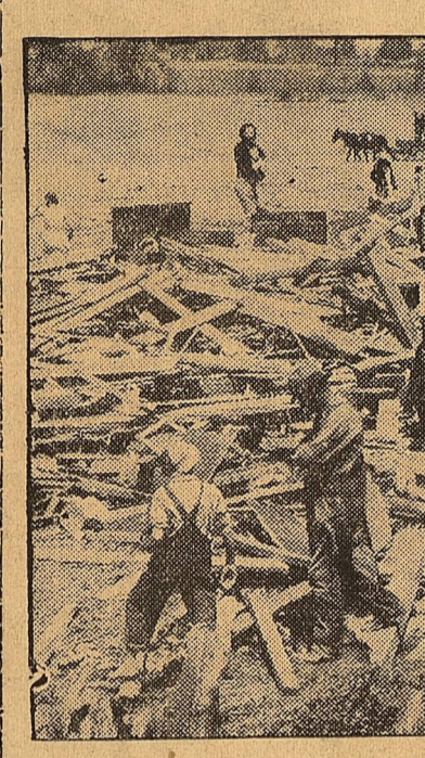
Above are the ruins of an old Southern home, owned by Mr. and Mrs. J. T. Dale of Millington, Tenn. Mrs. Dale, wife of a cousin of F. C. Dale of Midland,
