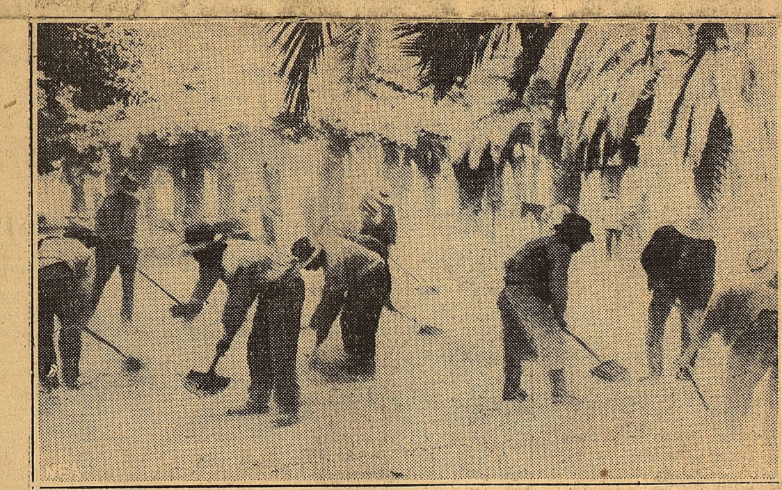
AS IF SHOVELING AWAY SNOW AFTER A STORM, workmen swarmed into the streets of Curico, Chile, to clear the pavement of tons of ash which fell upon the town from erupting Tinguiririca volcano, 75 miles away. Strange scenes like this were duplicated in scores of South American cities as craters along a 400-mile belt thundered into awesome activity, raining ash, smoke and gases over a widespread area. Note the blanket of volcanic ash upon branches of the trees.
