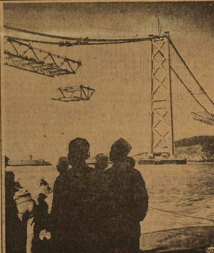
Swinging high above the waters of the bay, this huge fabricated section of the steel deck frame of the San Francisco-Oakland Bay bridge is being hoisted into place by traveling cranes. Moving far overhead, the cranes lift the section slowly upward from the barge on which it had been taken into the bay. By this engineering feat, all the framework for the two decks to carry nine lanes of vehicle traffic and two interurban tracks will soar into place, to be bolted and supported from the suspension system.
