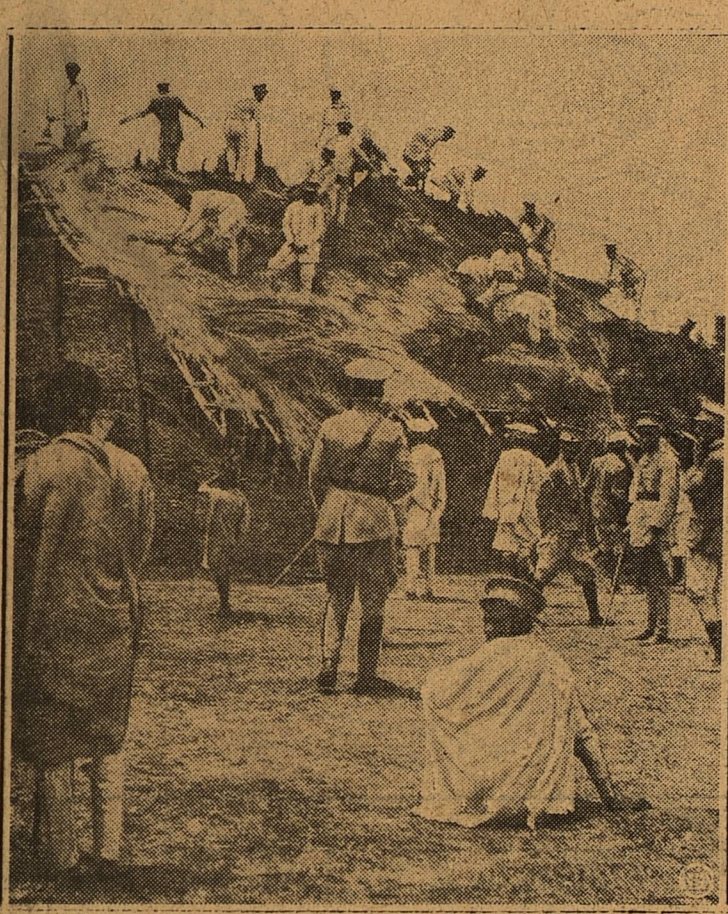
The Ethiopian army concentrating in the vicinity of Makale, is the most difficult of access in the far-flung war zone. Here is the first picture received in America from that remote area. It shows troops building a hut to house army headquarters.
