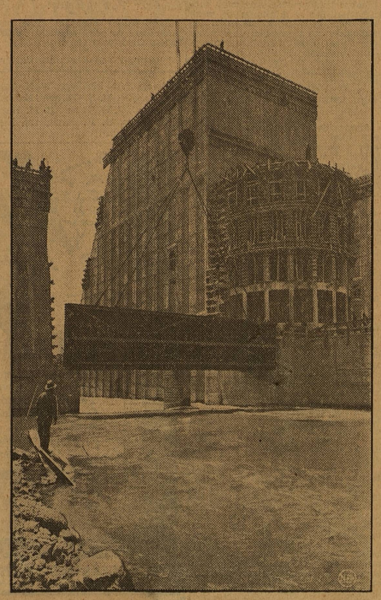
Despite the peril to President Roosevelt's entire program because of House opposition, work is going ahead at full speed in Norris Dam, key point of the mammoth TVA project in Tennessee.
