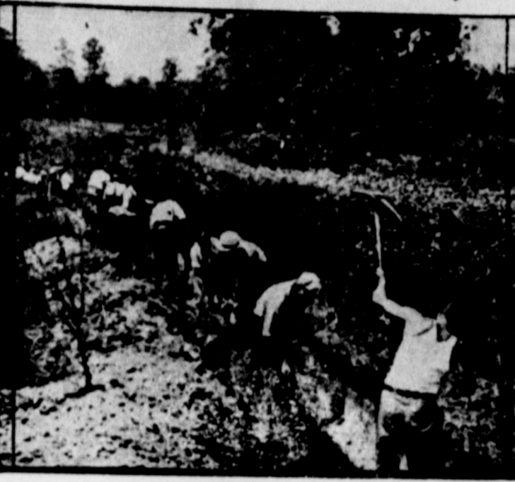
Workers are shown digging a water-line ditch, as work started on the housing project at Heighstown, N. J., where 200 assistance homes are being erected on a 1,270 acre plot by the Federal Housing administration.
