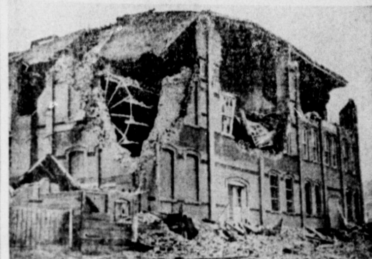
Helena, capital of Montana, was shaken by a series of earthquakes that continued through several days, and many buildings were wrecked or so weakened that they had to be torn down. The picture shows the damage done to the big plant of the National Biscuit company.
