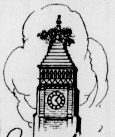
One or more Aspens have been growing on the Court House tower at Greensburg, Indiana since 1870. The present tree is 12 ft. high, rooting between blocks of limestone by T. D. Braden, Greensburg.
