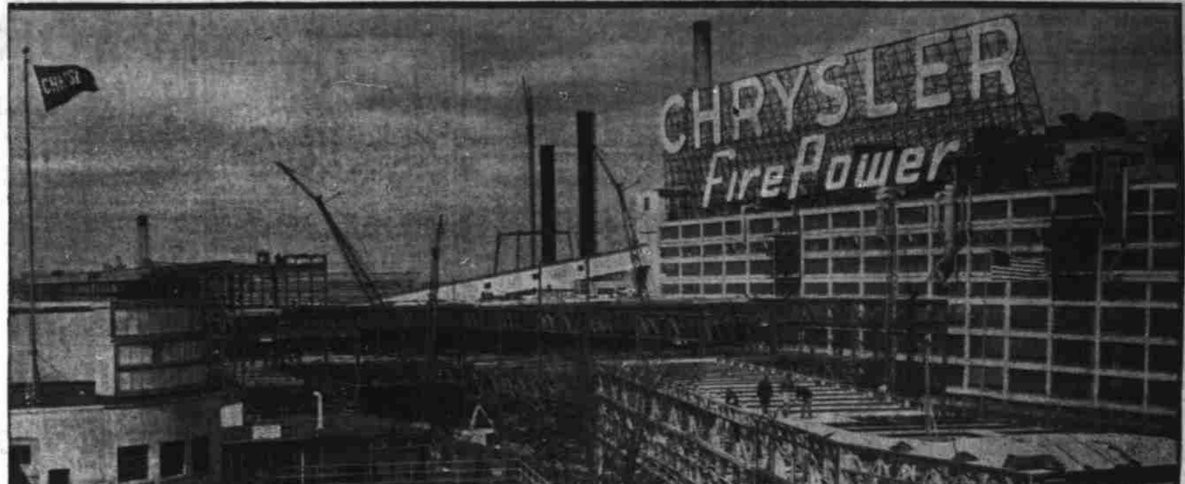
UP GOES CHRYSLER'S PRODUCTION MORE THAN 40% Here you see construction work proceeding on the new Chrysler production facilities which will add 687,000 square feet of floor space . . . including a 1 1/2-mile long continuous conveyor system, longest in the industry.
