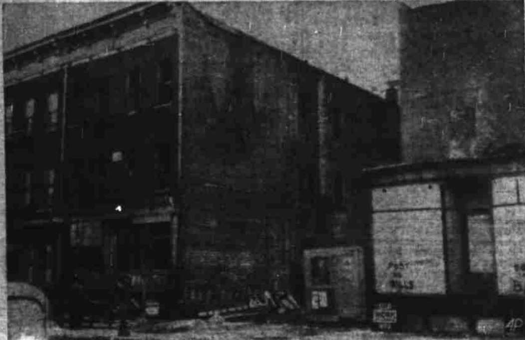
Embarrassed New York WPA officials reveal that the crew of workmen sent to raze a three-story building, at the owner's request, and in line with the city's improvement program, had—entirely by mistake—torn down the building next door, a three-story structure that had been abandoned. The vacant space above is where it used to be. The buildings had no street numbers, it was explained.
