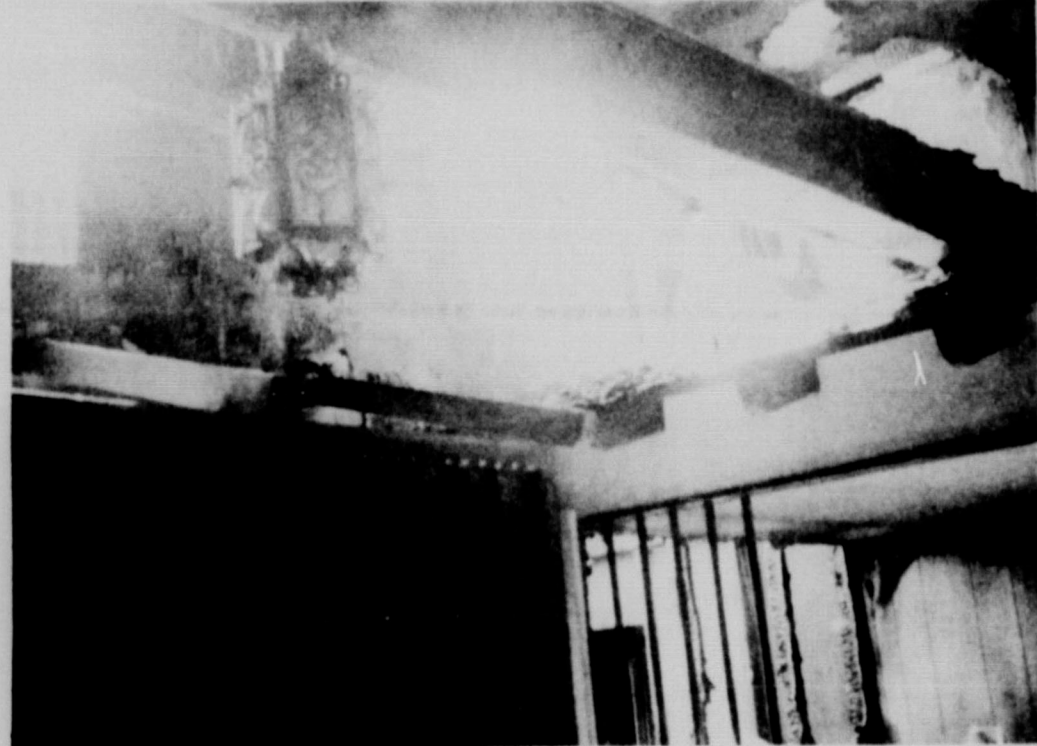
SUNLIGHT THROUGH THE ROOF shows the remains of the interior of the cafe early Tuesday morning. The photograph was taken at the cashier's station inside the building. Firemen spent several hours and several thousand gallons of water extinguishing the spectacular blaze.
