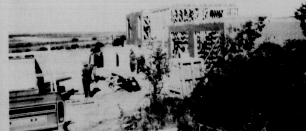
ANOTHER CONSTRUCTION SITE on the east hill is well under way. The split level project will be a clinic and living quarters for Dr. and Mrs. Don Carlisle. A Spanish style structure, the living quarters will be on a separate level from the medical clinic. The finished product will be white stucco with red tile roofing.
