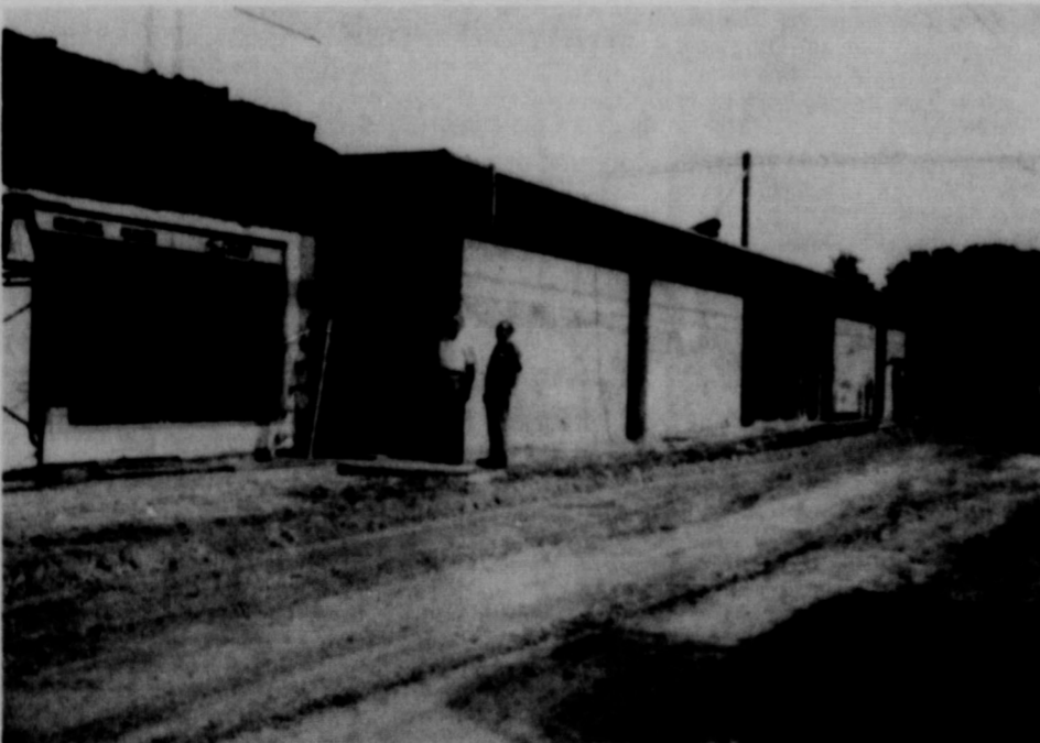
NEW ADDITION TO SOUTH TEXAS LUMBER CO. -- Work is progressing on the new addition to the company located at the intersection of highway 163 and I-10 in Ozona. The new addition will more than double the space of the present building. Here W. H. Whitaker looks over the expansion project with Arthur Madden, representative of one of the companies South Texas purchases materials from.
