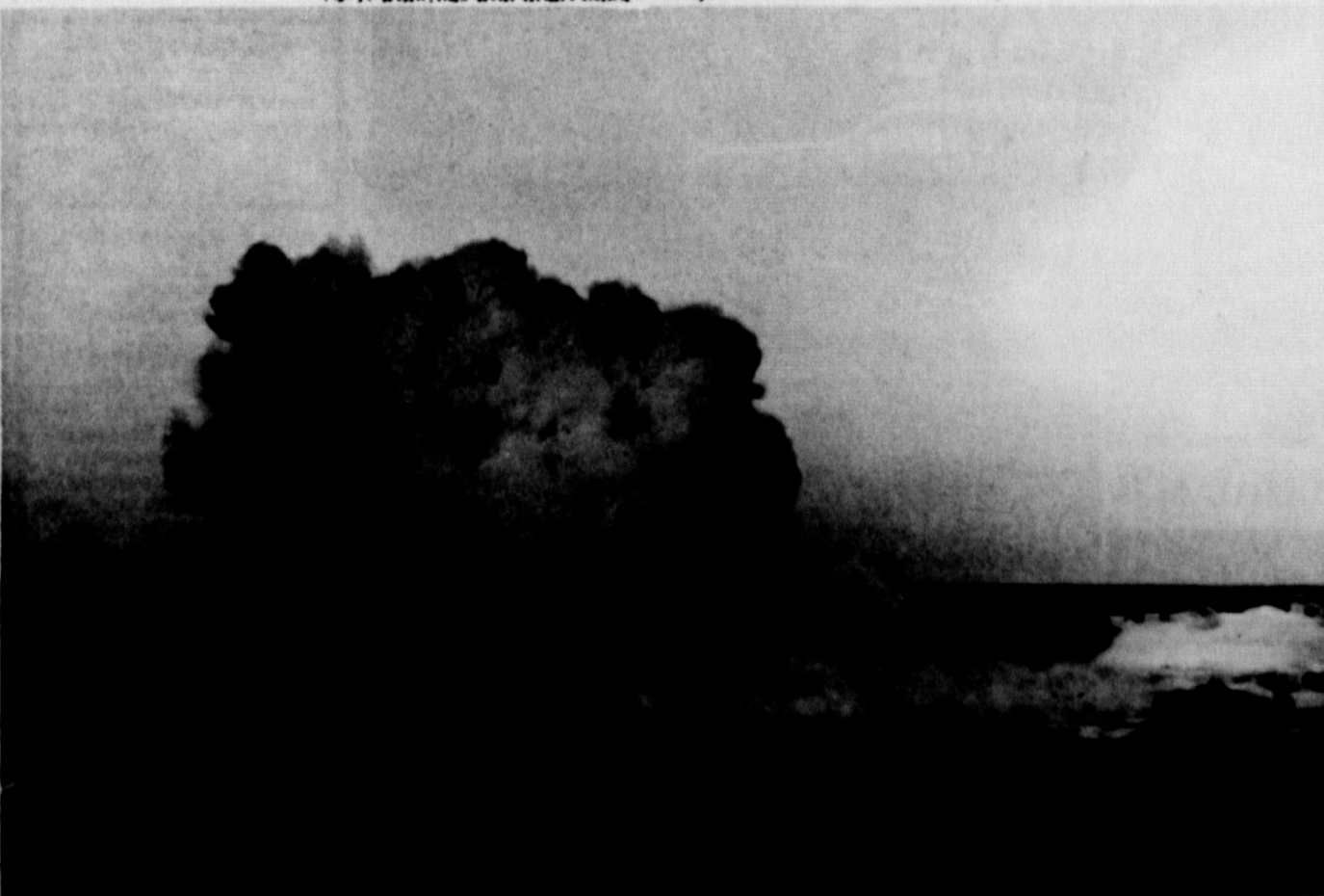
ONE OF THE BLASTS in the construction of Interstate 10 west of Ozona which is changing the face of the earth, along with the road machinery which is in constant operation. If the blasts
