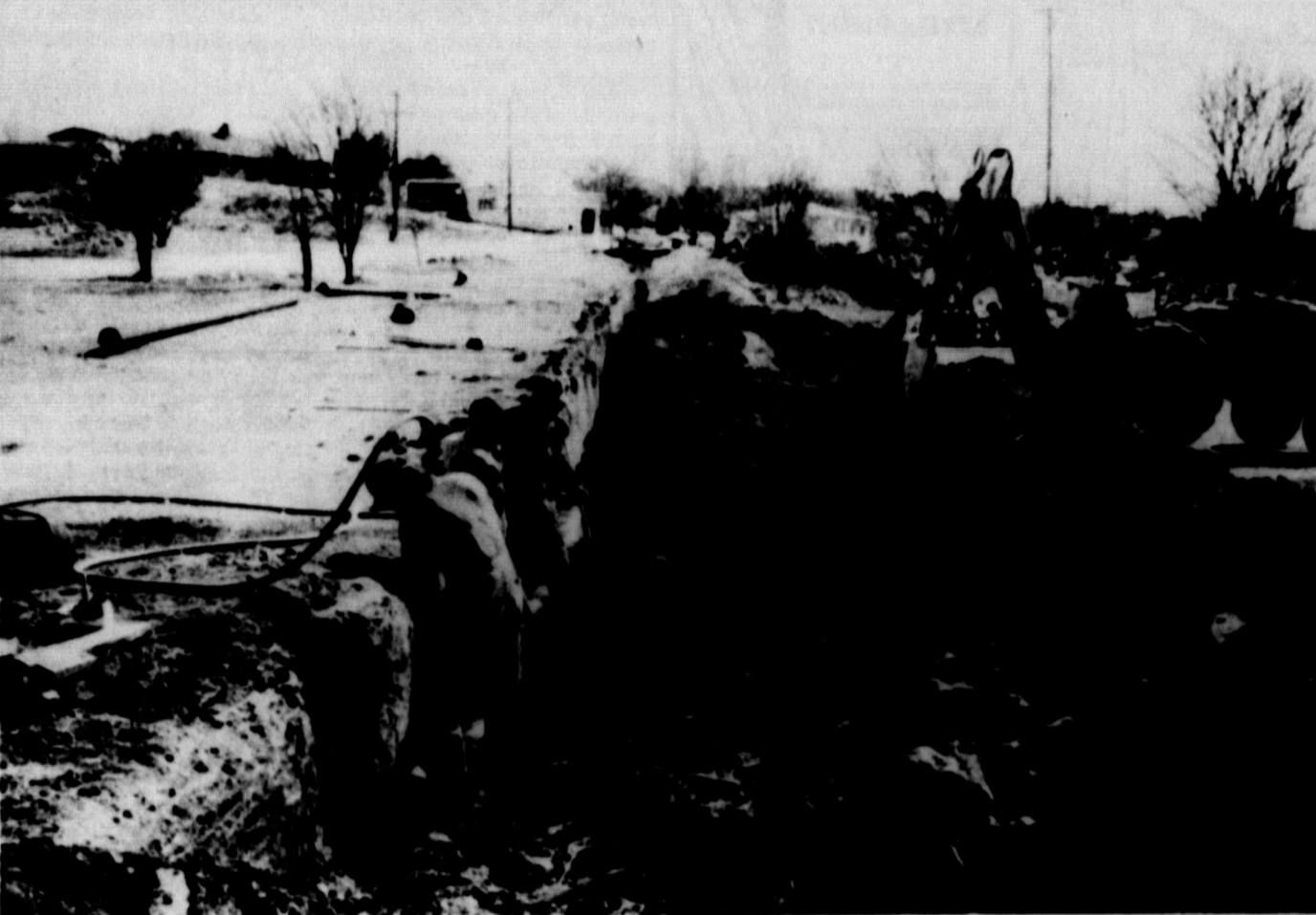
UTILITIES ADJUSTMENT FOR IS 10 -- Water district employees are hard at work re-routing water mains and sewer lines in lieu of construction of Interstate 10 through Ozona. Construction has been approved for the section which will extend from 0.8 mile west of State Highway 163, which runs through the center of Ozona, to 6.6 miles east of Ozona. All utilities must have relocation work completed by April 1. Bids will be called for in March for the approximately 6.9 miles of IS 10.
