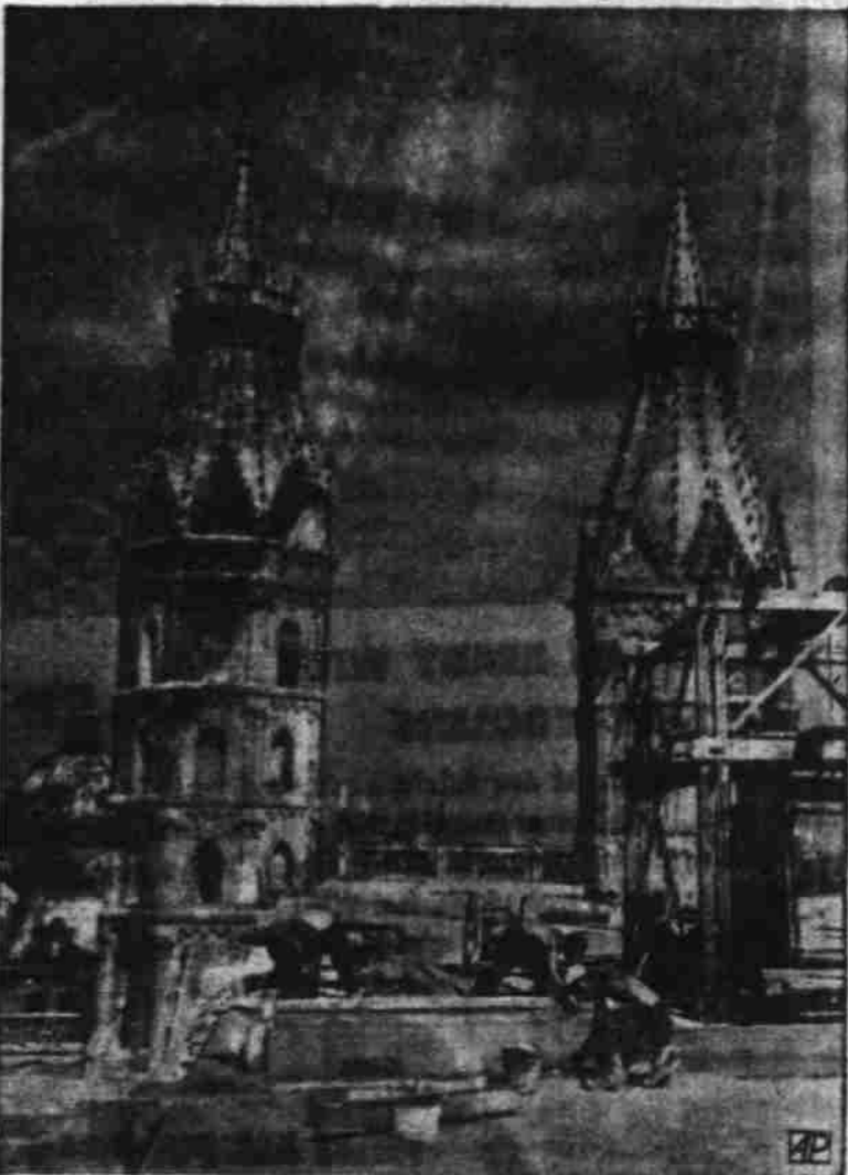
CATHEDRAL REPAIRS — Workmen repair the roof of the bomb-damaged Cathedral of St. Stephen in Vienna—one of the city's most beautiful buildings. In background are two Heiden Towers which decorate the front of the roof.
