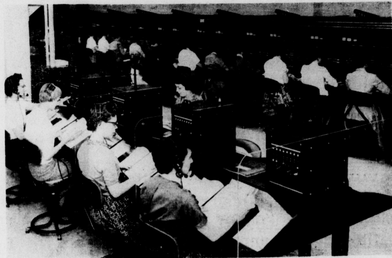
OZONA'S LONG DISTANCE CALLS go through the modern 54-position switchboard in San Angelo. Operators shown above can dial direct throughout the United States and Canada. Information positions are in the foreground.
