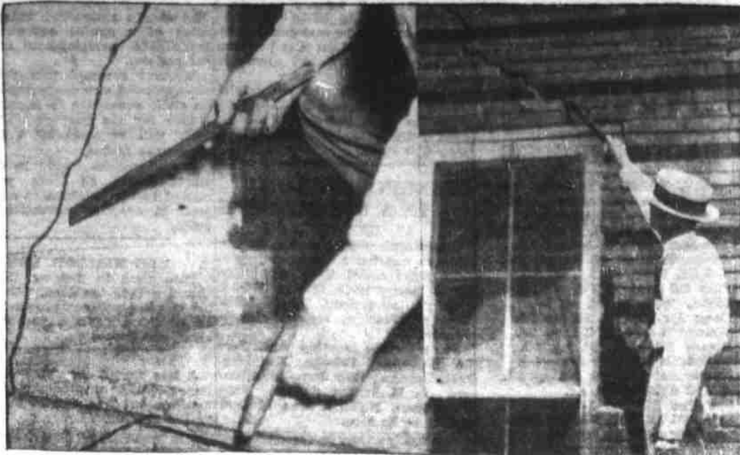
Some of the reasons why the school board deemed it wise to condemn a section of the senior high school are shown in the above photograph. At the left are shown cracks appearing at a stairway adjacent to
