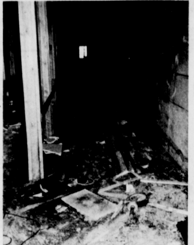
The American National Bank is in the midst of an extensive remodeling (Photo by Linda Haynes)
