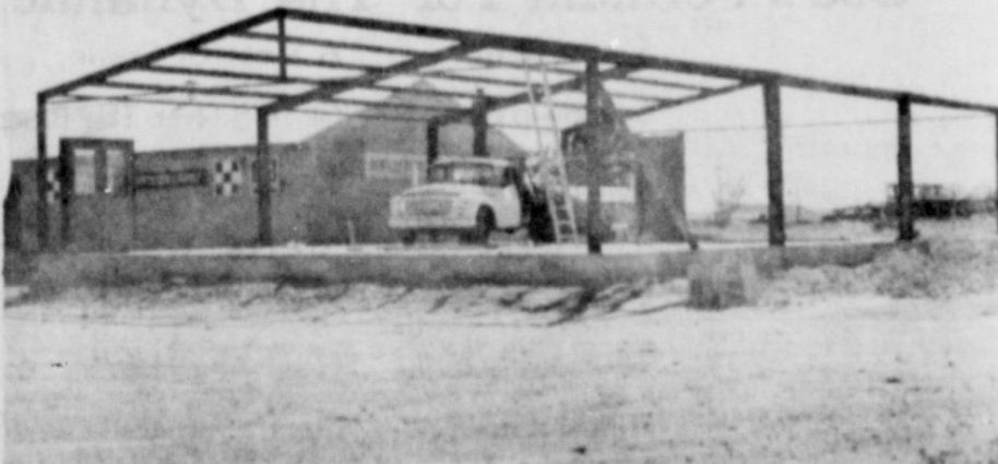
Bentley Fertilizer Co. has a new building under construction. The structure will house an office and additional feed and fertilizer storage and will be connected to the present feed building. Work began about a month ago, and the Bentleys are hoping for an Oct. 1 completion date. (Staff Photo by Lisa Patman)
