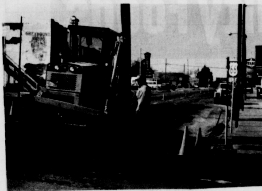
HIGHWAY DEPARTMENT CREWS reworked the backtop on Interstate 40 near downtown McLean. The pavement was laid last year over the brick streets, but had become "wrinkled" by large trucks stopping at the stop light. (Photo by Linda Haynes)
