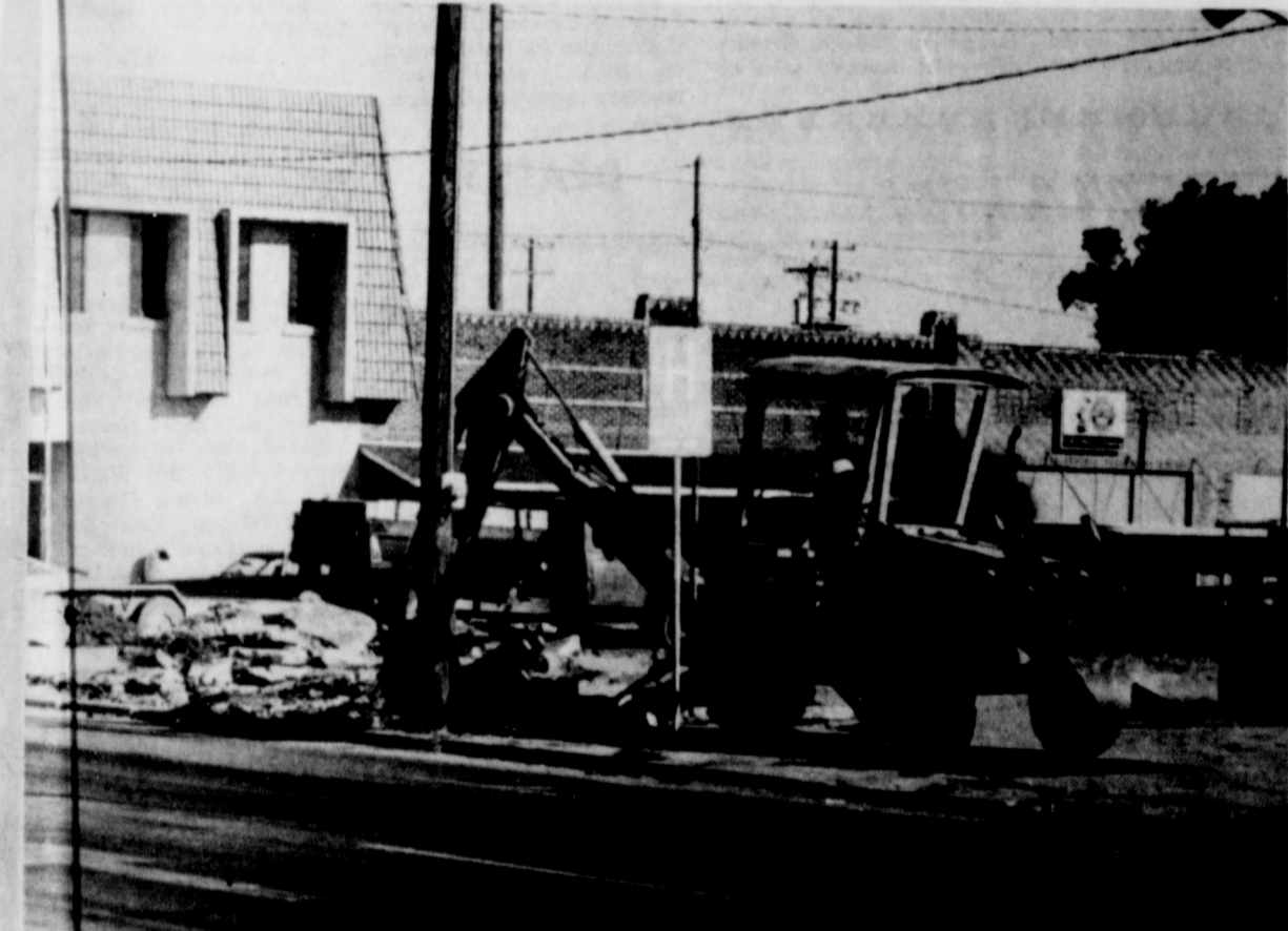
CONSTRUCTION BEGAN TUESDAY on the downtown park for McLean. Britt Hathaway, Jim Barker, and Danny Rice are doing the preliminary work for the park which will eventually have a gazebo, a fountain, and parking areas for downtown. [Photo by Linda Haynes]
